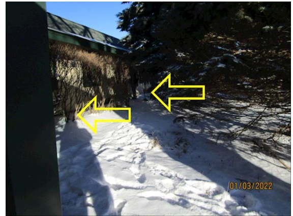
Grading / Drainage: Negative
