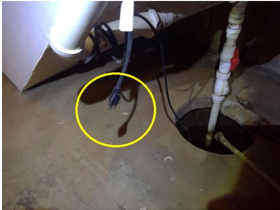
SUMP/SUMP PUMP: IO
