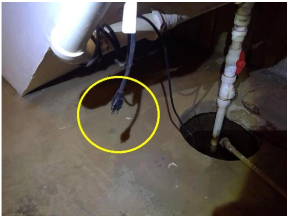
Sump/Sump Pump: IO
