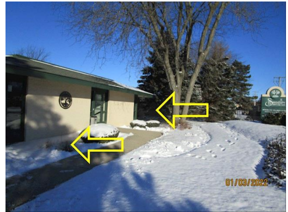
Grading / Drainage: Negative
